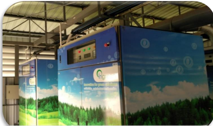
Ozone System, PWA - Chachoengsao
