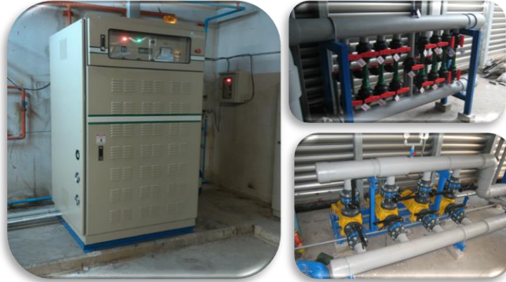
Ozone for Cooling Tower, ESPLANADE
